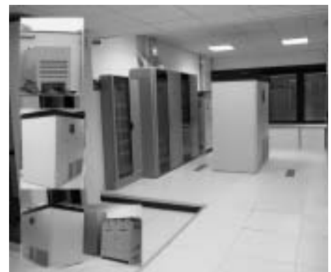
Data Center Milan, Italy
