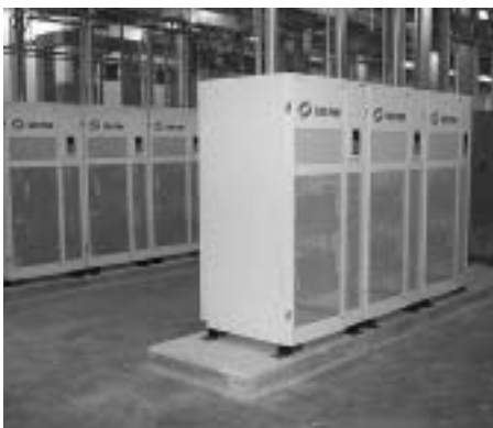
Internet Data Center Atlanta
